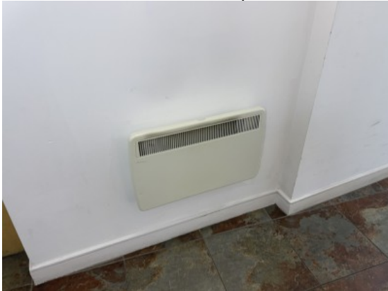
Hardwired wall mounted heaters noted in common parts
