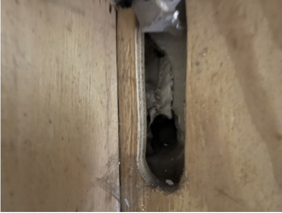
Missing ironmongery/ holes noted to service cupboard doors which could compromise integrity in the event of a fire
