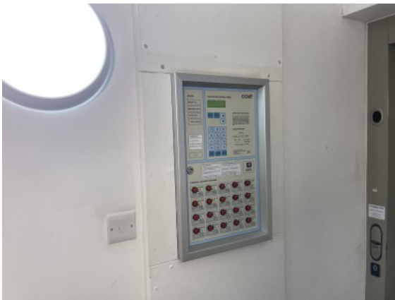
Smoke vent system - control panel
