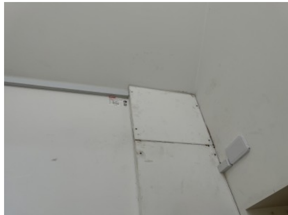
Service riser not constructed in fire resistant materials
