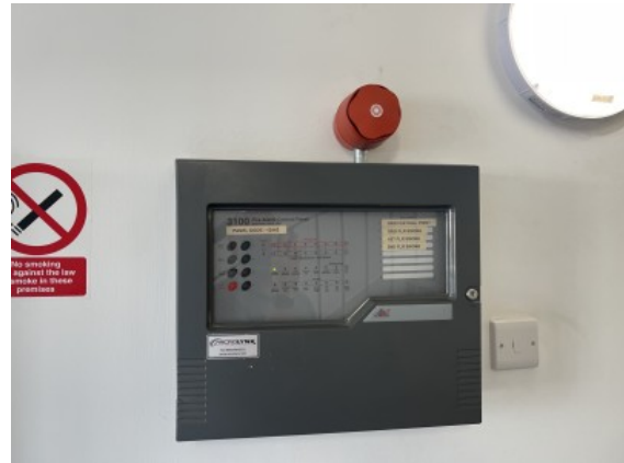
Fire alarm panel in common parts
