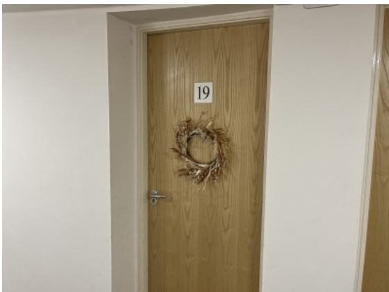
Combustible materials affixed to private flat entrance doors
