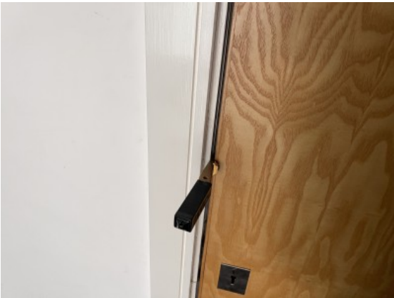
Gaps in excess of 4mm between service cupboard fire doors and respective frames and/or abutment joints.
