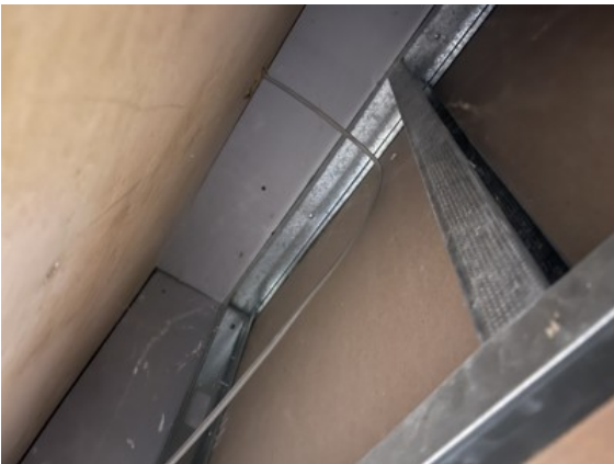
Incomplete compartmentation in riser cupboard
