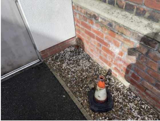
28-64 - Evidence of discarded smoking materials adjacent to building perimeter
