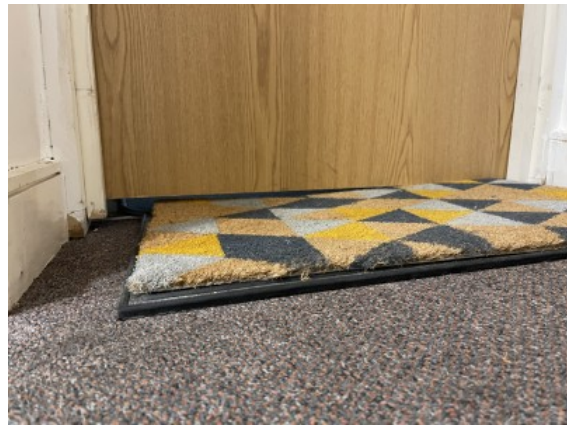
Gaps in excess of 10mm above floor finish to base of flat entrance fire door
