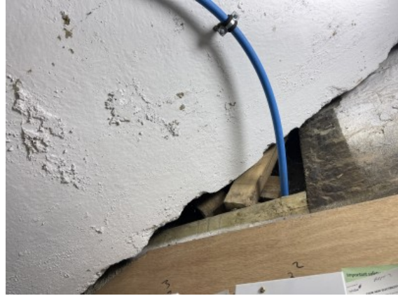
Incomplete fire stopping of cable/pipe penetrations in electric intake cupboard
