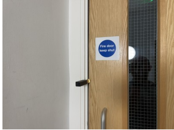
Gaps in excess of 4mm between cross corridor fire doors and respective frames and/or abutment joints.
