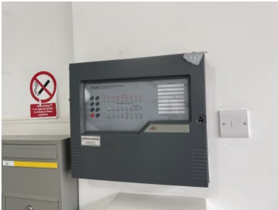
Fire alarm panel in common parts
