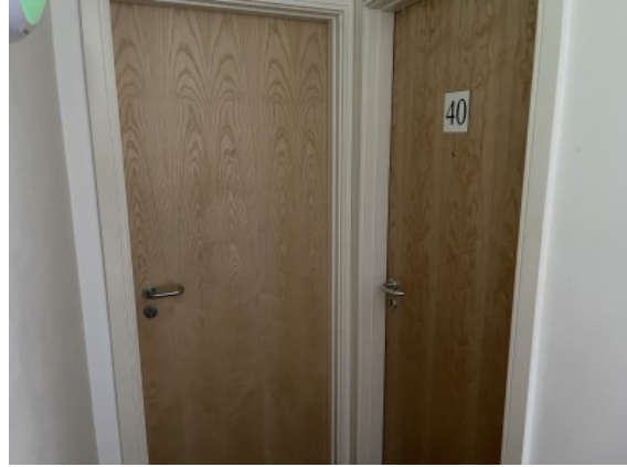
Retrospectively installed flat entrance door - FD rating unknown.
