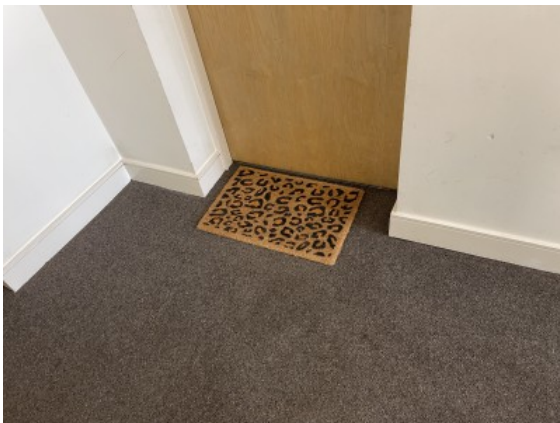
Private flat entrance door mats noted on escape routes
