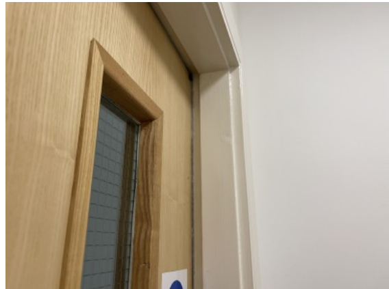
Example of cross corridor fire door not closing into frame rebate of its own volition
