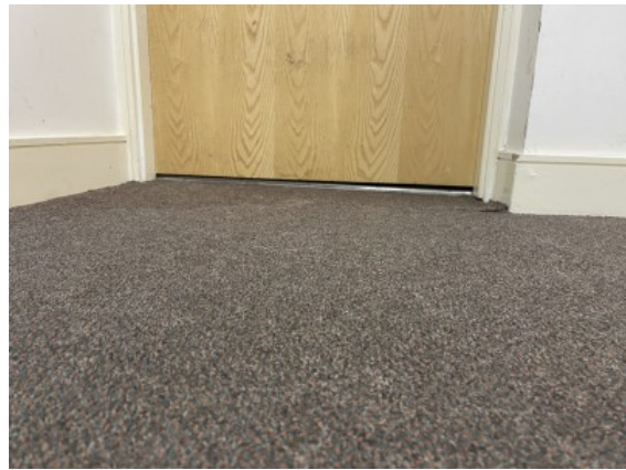
Gaps in excess of 10mm above floor finish to base of flat entrance fire door
