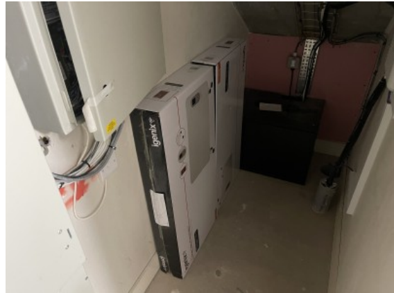
Combustible materials noted in service cupboards
