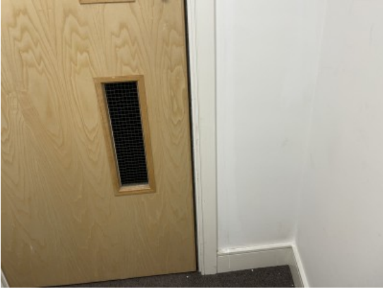
Gaps in excess of 4mm between cross corridor fire doors and respective frames and/or abutment joints.
