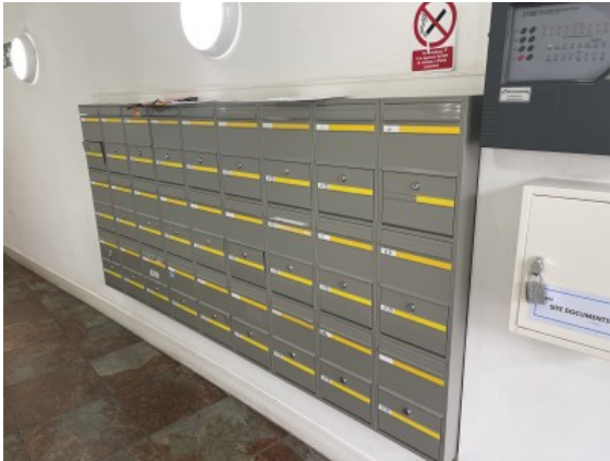
Internal letterbox system installed in common parts
