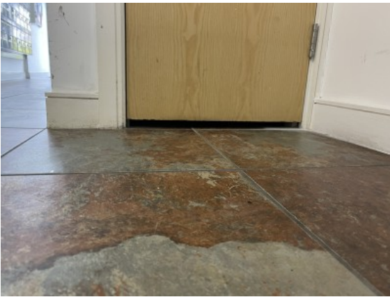
Gaps in excess of 10mm above floor finish to base of service cupboard/riser fire door
