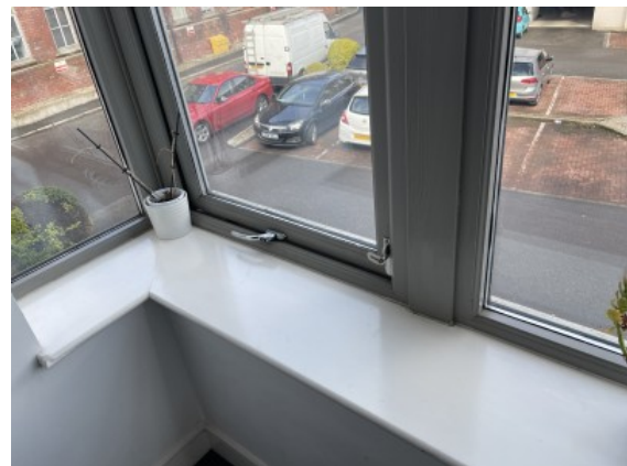
Key operated window restrictors noted to apertures off escape routes
