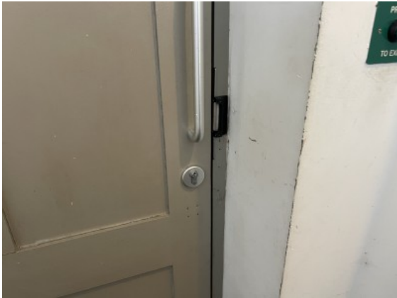
77-78 - key operated barrel lock to the final common egress door
