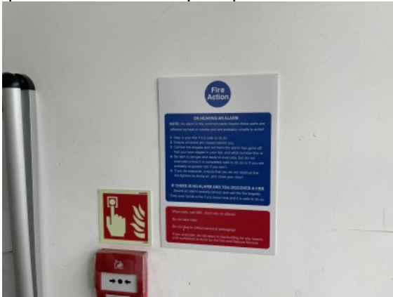
Incorrect simultaneous fire action notices present in common area
