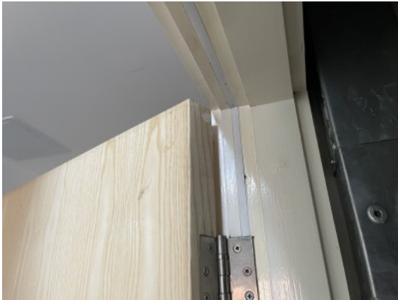
Absence of cold smoke seals to service cupboard fire doors
