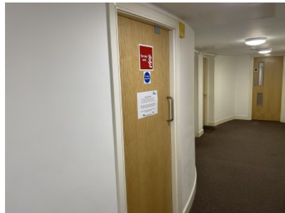
Smoke vent system - AOV
