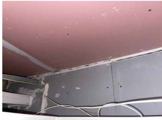
Incomplete compartmentation in common ceiling voids
