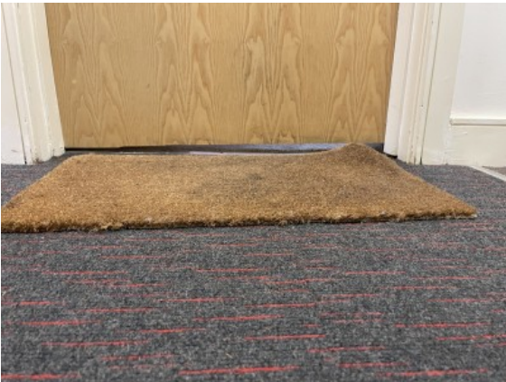
Gaps in excess of 10mm above floor finish to base of flat entrance fire door
