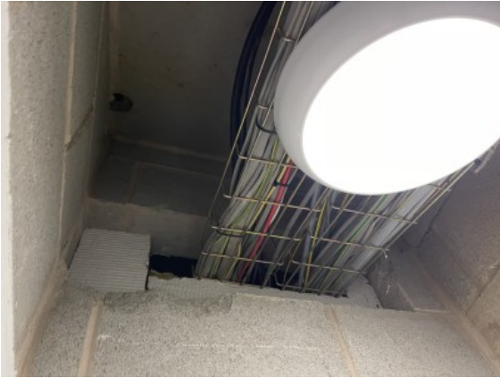
Incomplete compartmentation in riser cupboard
