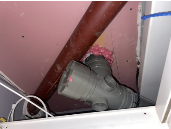
Incomplete compartmentation in common ceiling voids
