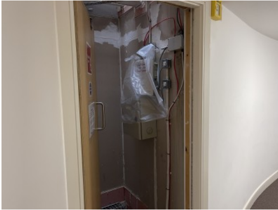
Example – smoke shaft door held open
