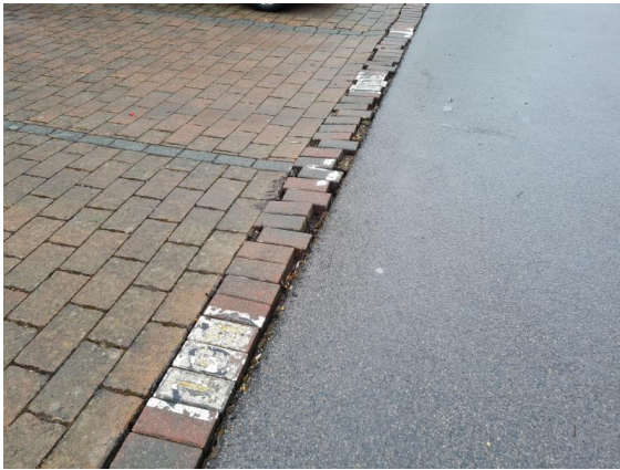
Examples of raised and loose block paving
