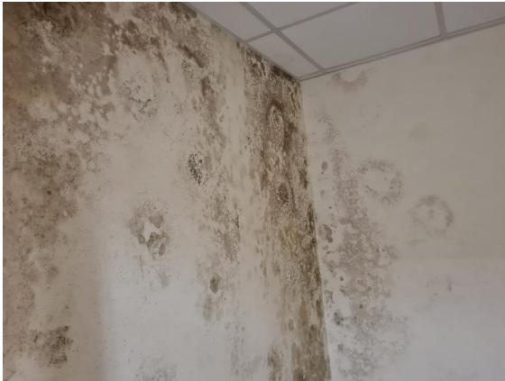
Damp found in cupboard outside 103
