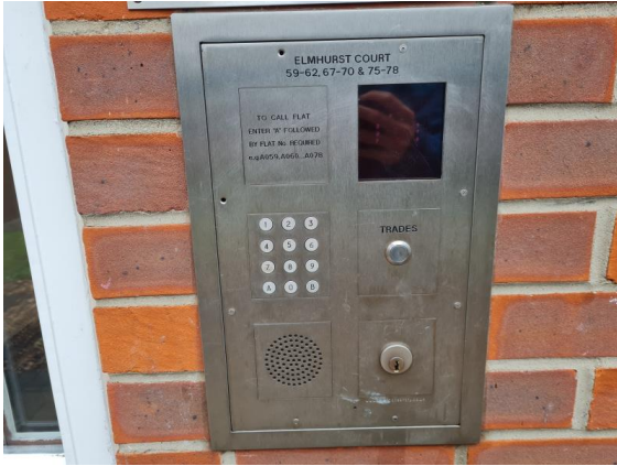
Example of occupier operated intercom system installed
