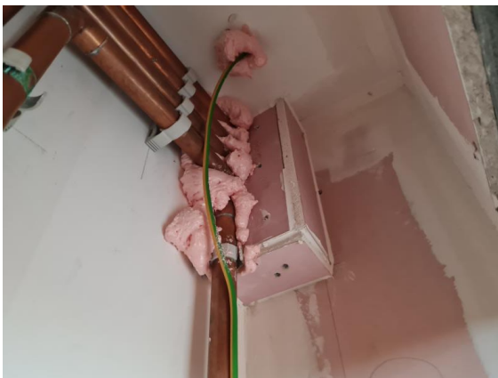
Excessive use of fire foam
