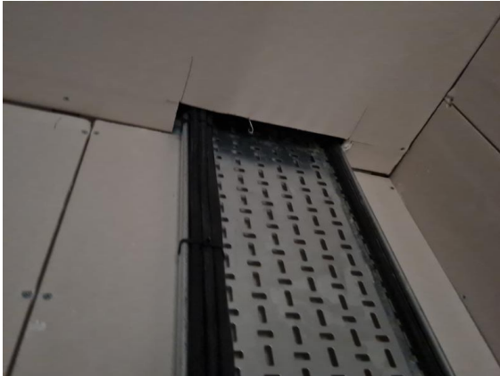
Example of lack of fire separation
