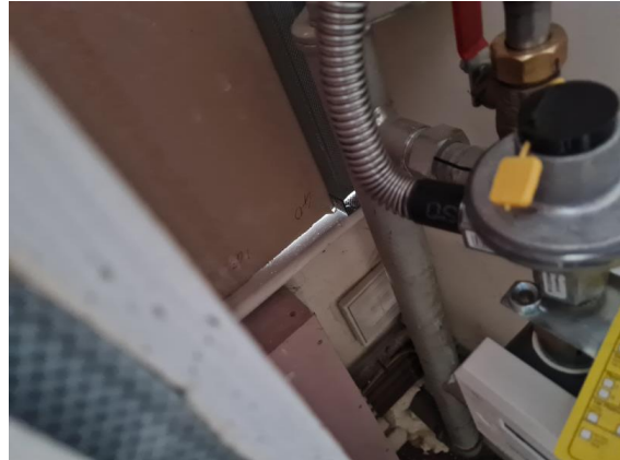
Example of lack of fire separation
