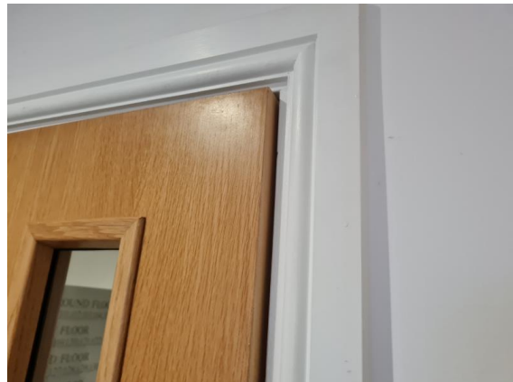
Example of cross corridor door not sat in frame
