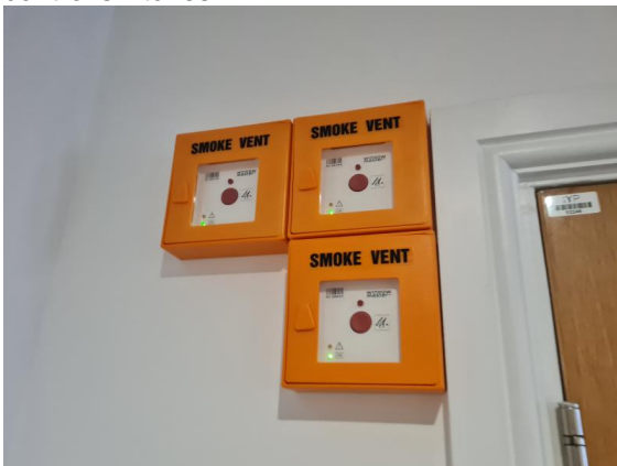
Example of smoke vent controls
