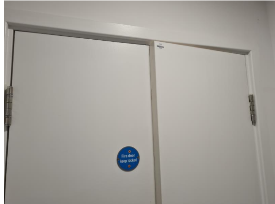
Example of doors out of 4mm tolerance
