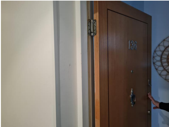
Flat entrance door only fitted with 2 hinges not 3
