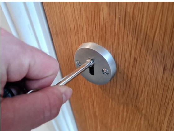
FB keys cant get into locks to lock doors
