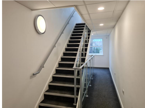
Example lack of fire escape route signage
