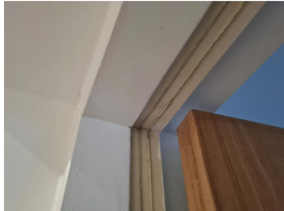
Flat entrance door fitted with intumescent strips but no self closer
