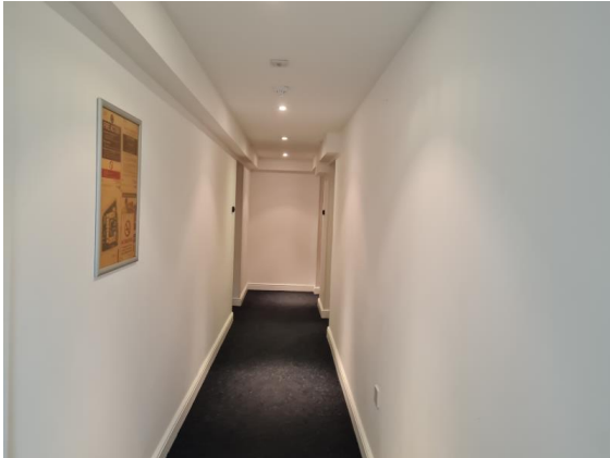
Example lack of fire escape route signage
