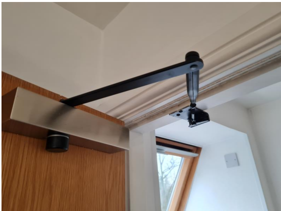
Cross corridor doors are fitted with self closing devices and intumescent strips
