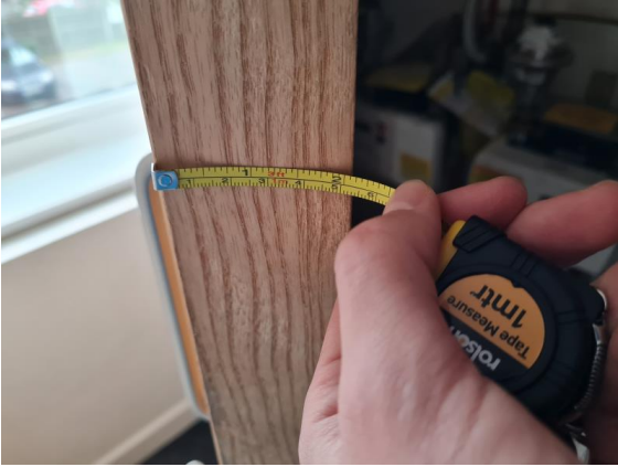
Example of FD60 fire doors used on service cupboards
