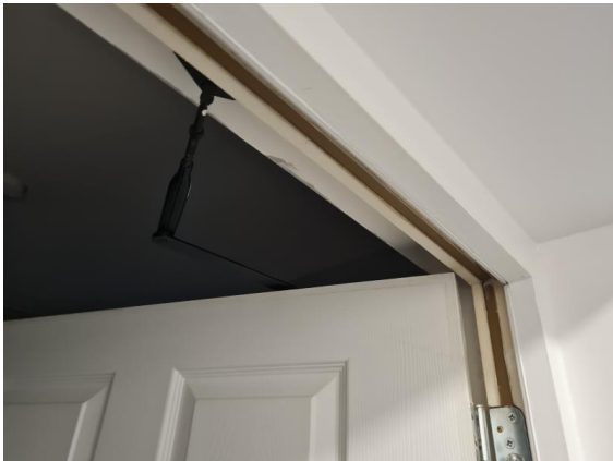
Flat entrance door fitted with self closing device
