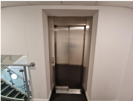
Lack of Lift signage
