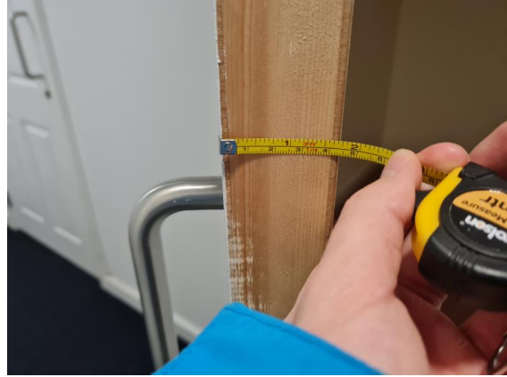
Example of FD30 fire doors used on service cupboards
