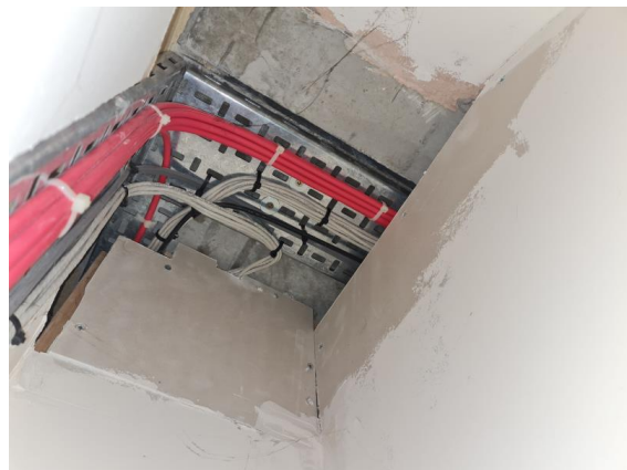
Example of lack of fire separation
