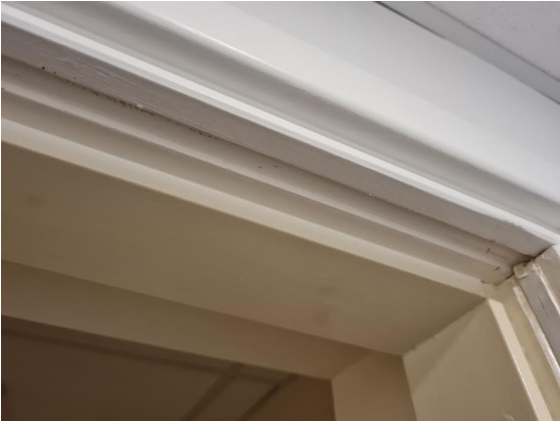
Lack of intumescent strips example on service cupboards
