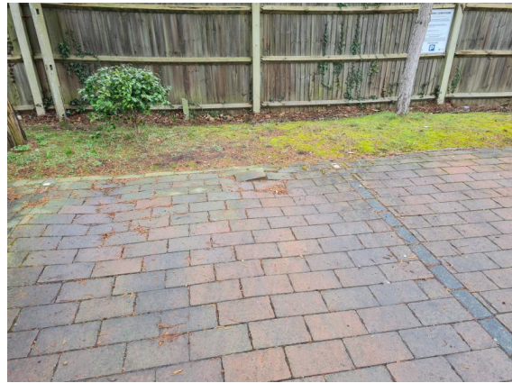
Examples of raised and loose block paving
