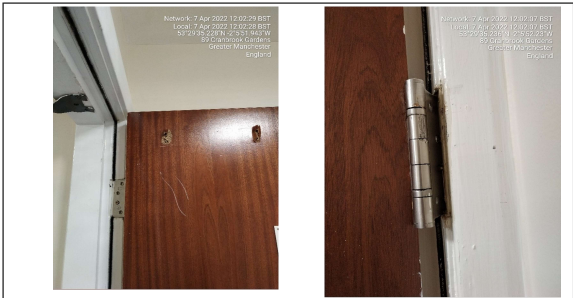
Photo No. 2 Lobby door into 93/94 Significant damage to door and frame
