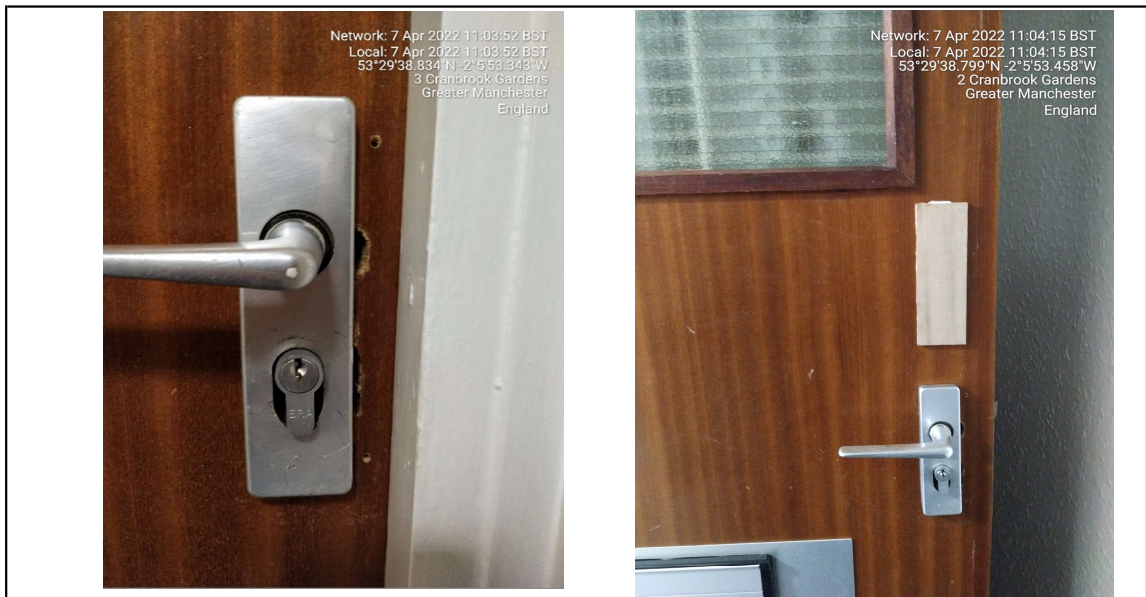
Photo No. 1 Flat 24 Hole in Fire door around handle Previous damage repair
